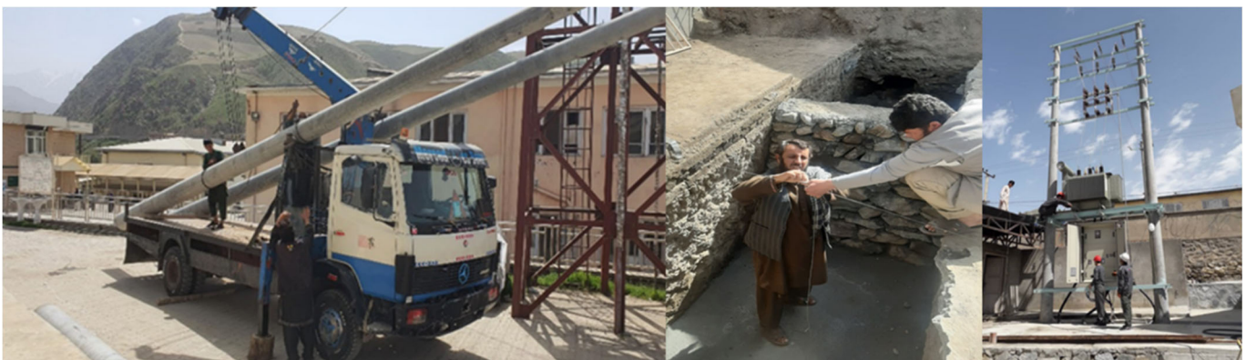
Installation of a 1000KVA Transformer and connection to grid of the AKHS,A- Faizabad Hospital, 2022.
