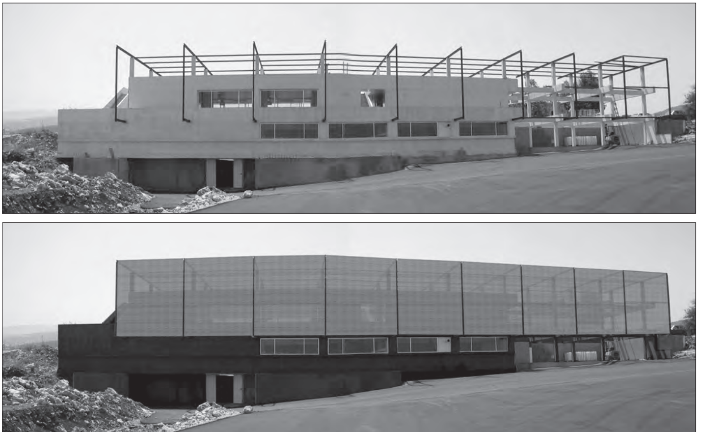
Fig. 10: Olive-Oil Press, view of the north elevation during construction, and a reconstructed image of the elevation showing the applied bamboo skin.
