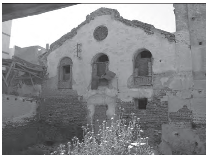
Fig. 20: Ginning mill next to the Tarbush Factory, eastern main facade of the truss-roofed workshop building.
