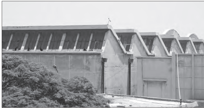
Fig. 67: al-Shirka al-Ahliyya, new dye works for cloth, 1960s extension with north-light saw-tooth roof.
