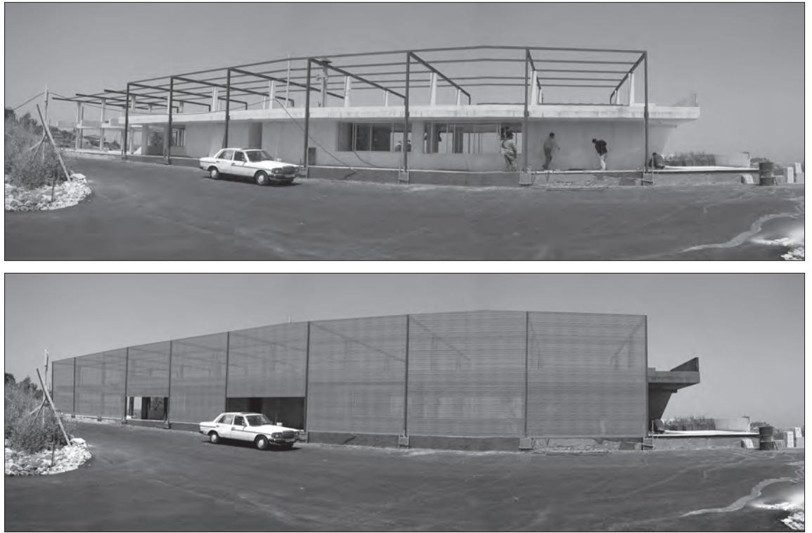
Fig. 9: Olive-Oil Press, view of the south elevation during construction, and a reconstructed image of the elevation showing the applied bamboo skin.
