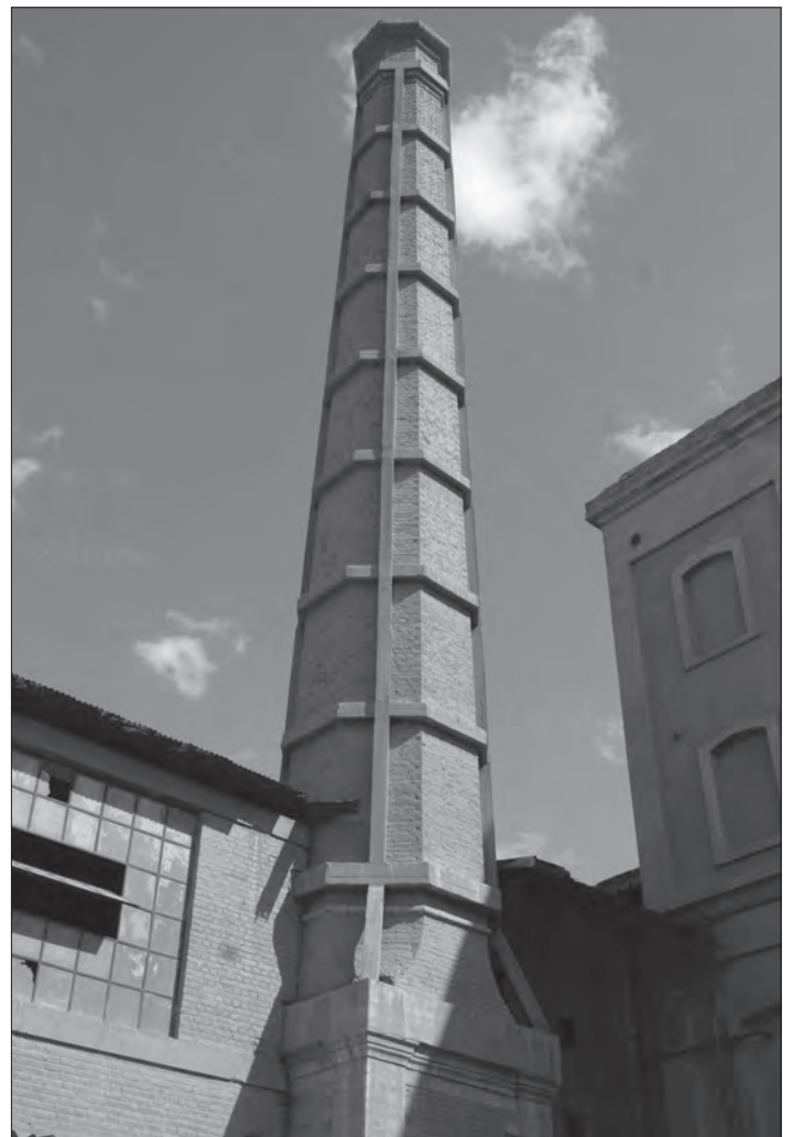
Fig. 30: Salvago Ginning Mill, chimney with the subsequently-added concrete bracing.
