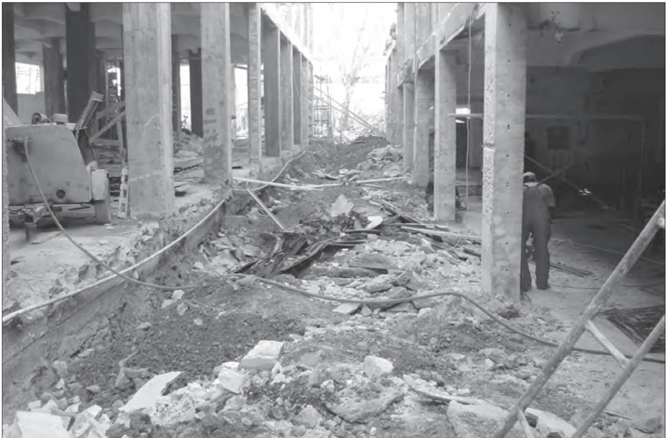
Fig. 15: BU Campus, the narrow street separating the two buildings during the construction process.
