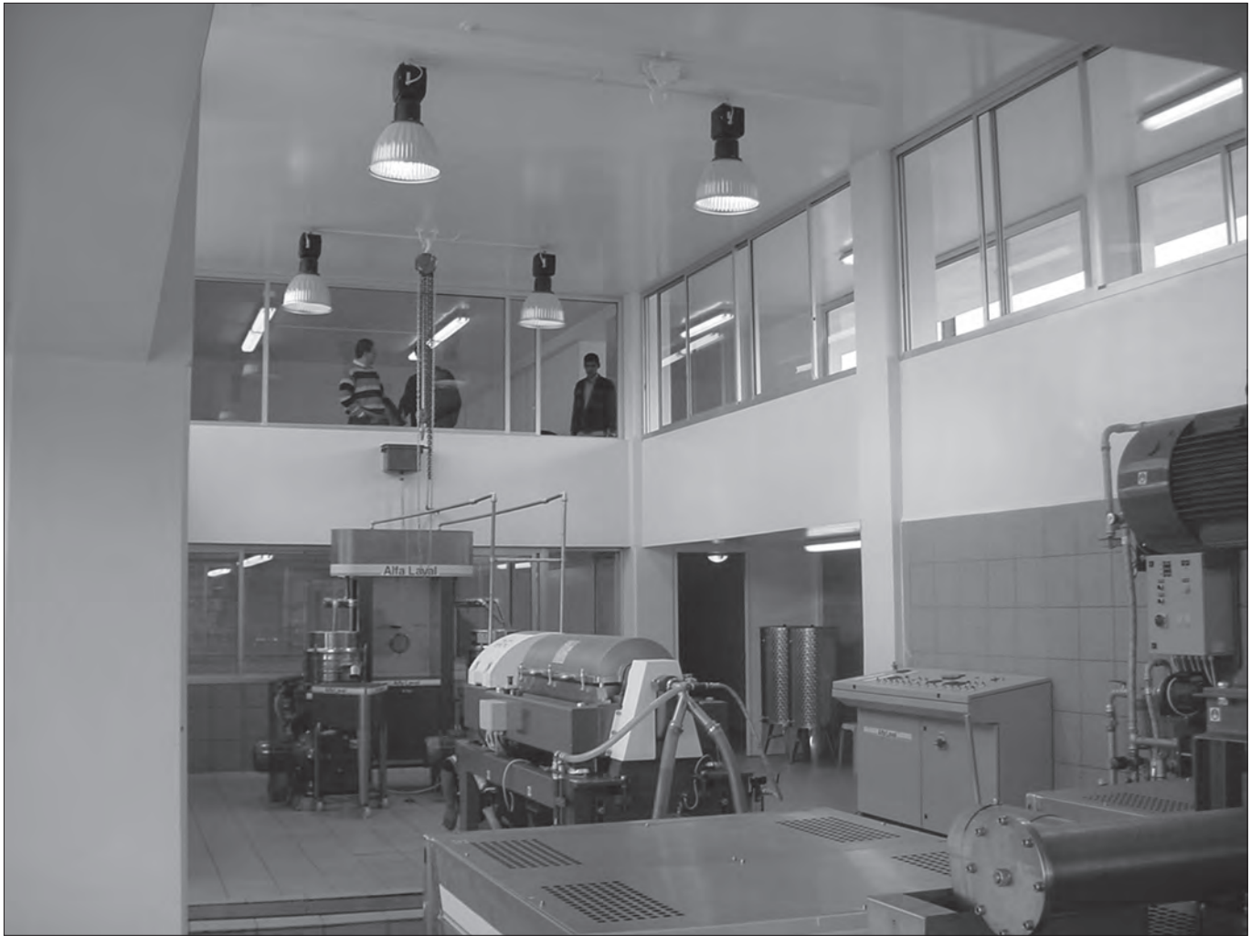
Fig. 11: Olive-Oil Press, interior view the olive-oil press machinery and the second-floor viewing platform.
