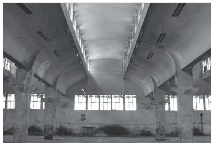
Fig. 65: al-Shirka al-Ahliyya, new dye works for cloth, interior view showing cantilevered shell roof.
