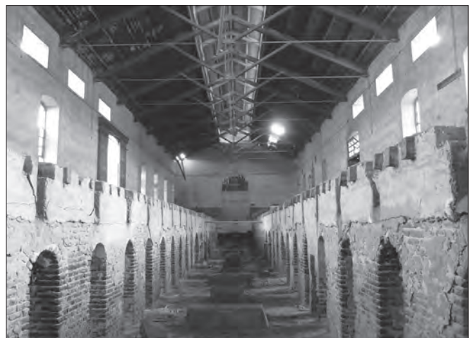
Fig. 28: Salvago Ginning Mill, main ginning hall, interior view; the main floor has been removed, rendering the substructure that used to support it visible.
