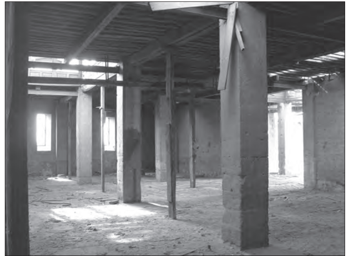
Fig. 7: Citadel Arsenal, workshop hall facing the gun foundry, view of timber roof on stone pillars.
