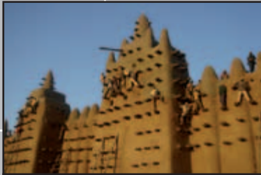
Culture: In Djenné, AKDN has restored the Great Mosque as part of its Earthen Architecture Initiative.
