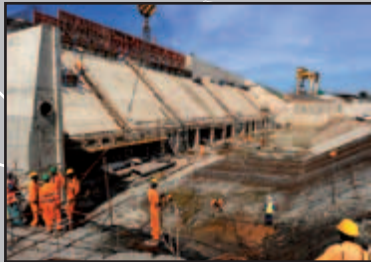
Industrial Promotion: The US$ 770 million Bujagali Hydroelectric Power Project in Uganda is one of the largest independent power plants in sub-Saharan Africa.
