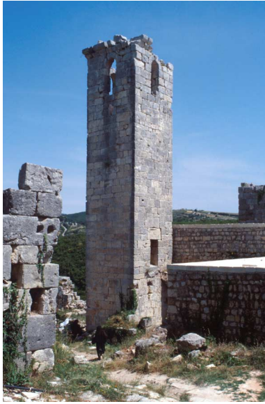
The minaret: An earthquake had broken the top of the minaret apart. To ensure structural stability, the top
