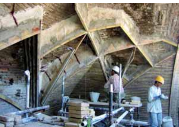
Local craftsmen restoring the vault of the historic Chahar suq cistern in the old city of Herat.
