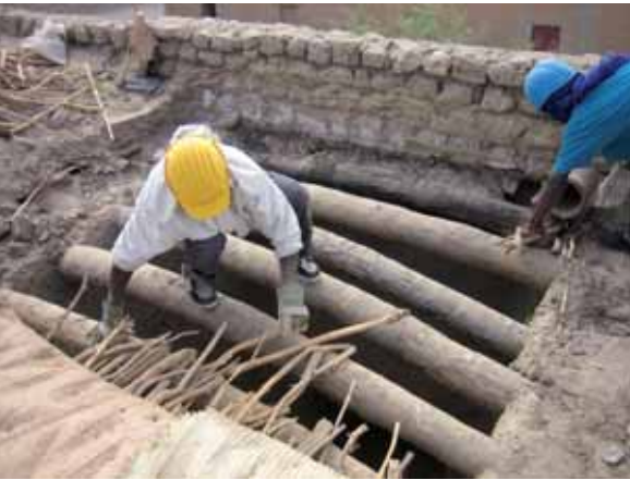
In Mali workers replace roof timbers as part of housing improvement programmes.
