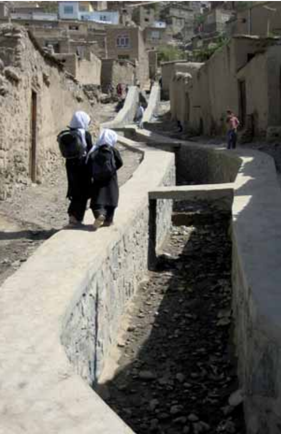
Improved drainage in the informal settlements above the garden of Babur in Kabul.
