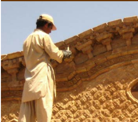
Embossed pattern bricks, typical of historic houses in Herat, have been restored on site by local craftsmen
