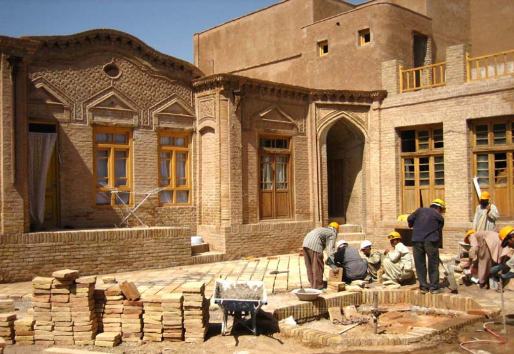
View of the restored Akhawan house during the paving of the courtyard
